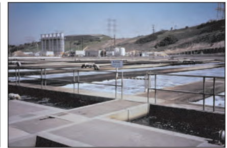
Martin Sheaves are use in the aeration tanks.
