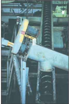
Martin Shaftless screws are used for removal of sludge which is hauled off to landfill or incinerated. In addition Martin V-Belt Sheaves are used on the motors.
