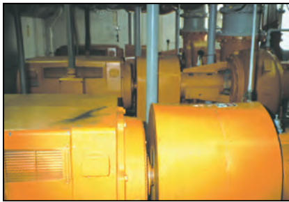
Martin Couplings and Sheaves can be found in the pumps at the lift station and in various other areas to move water from station to station.
