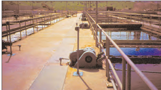
Martin Engineered Class Sprockets are used in the settling tanks.
